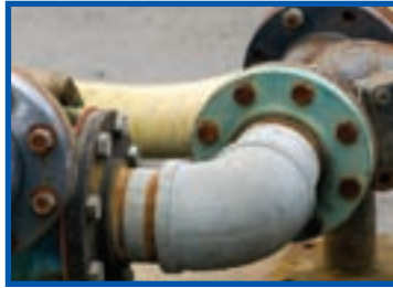
Compressed asbestos gaskets to pipework flanges
