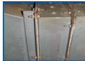
Chrysotile rope seals to flanges of ductwork
