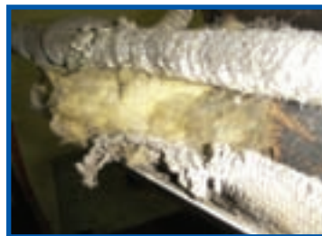
Chrysotile rope lagging to pipework
