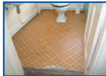
Chrysotile backing to linoleum floor covering
