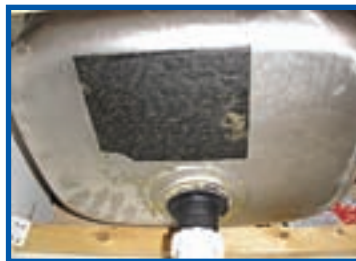
Chrysotile-containing bitumen pad to underside of sink
