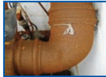
Chrysotile rope to metal boiler flue
