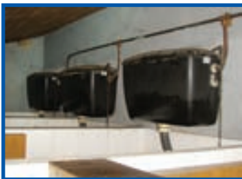
Asbestos-containing shires lynx toilet cisterns
