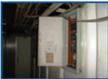
AIB to fuse panel door
