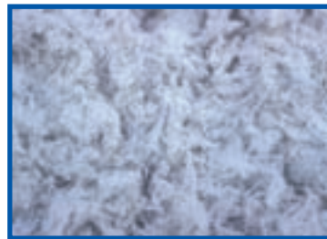
Asbestos loose lagging under floorboards, disturbed by plumbers
