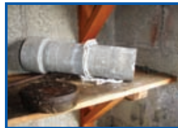
Chrysotile rope to asbestos cement flue pipe
