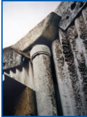
Asbestos cement barge boards and downpipe
