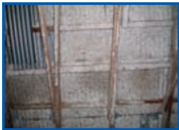
Asbestos spray coating to metal corrugated roof
