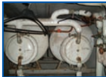
Thermal insulation to calorifier
