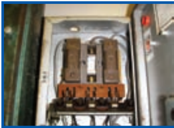
Chrysotile flash guards in old fuse box
