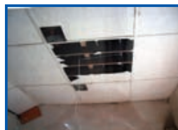
Damaged AIB ceiling panels
