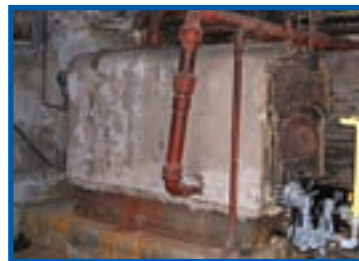
Thermal insulation to boiler
