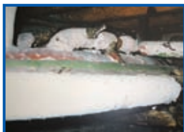
Composite asbestos lagging to pipework in very poor condition
