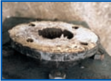
Exposed chrysotile-based compressed asbestos gasket to flange
