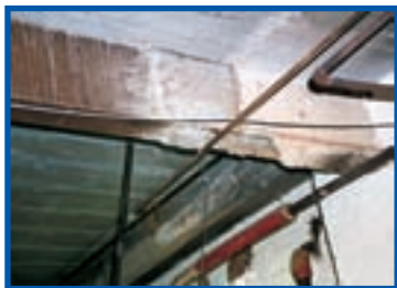
Asbestos spray coating to Rolled steel joist
