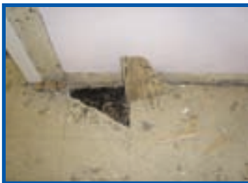
Chrysotile-based floor tiles and chrysotile containing adhesive
