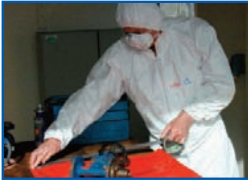
Use of tape and polythene sheeting to protect a work area before cleaning asbestos gaskets from a valve
